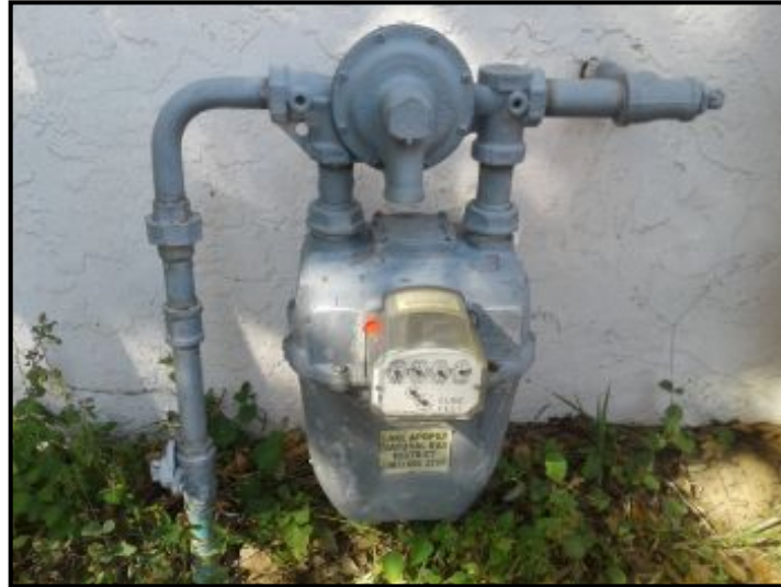
Main gas shutoff
