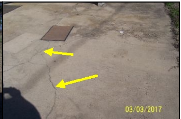
Some cracking of patio deck, seal cracks
