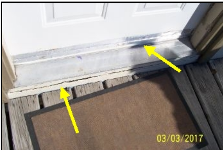
front door needs weather proofed and sealed
