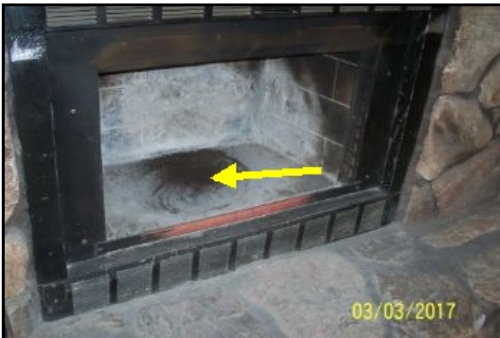
flue had some soot fall when damper operated
