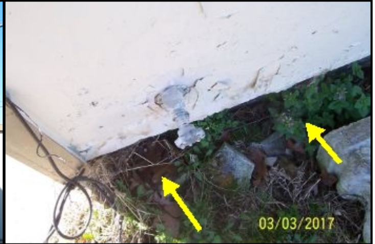
paint chipping from siding, negative grade toward house
