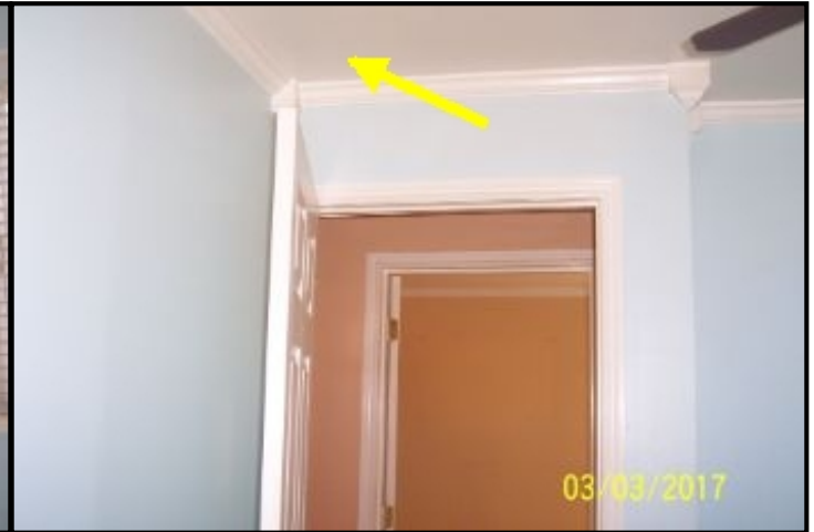
no smoke alarm
