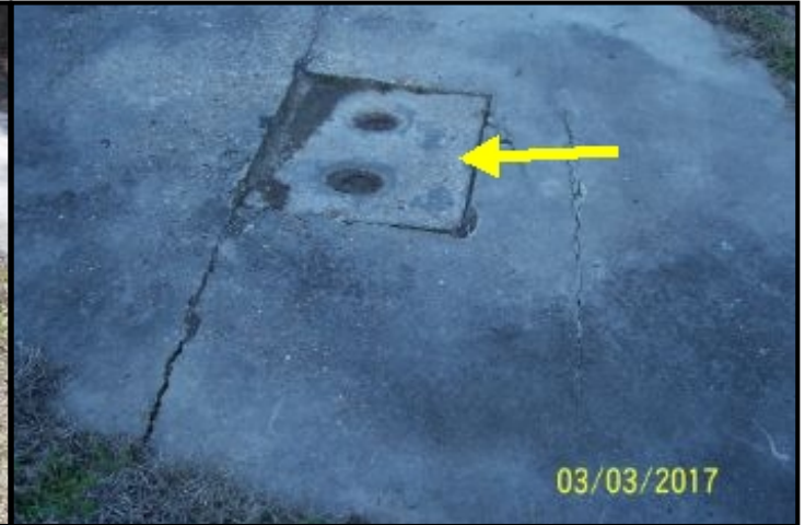
septic tank cover, should be covered with soil and lid extension
