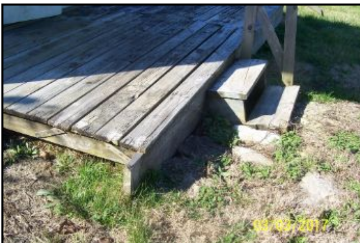
wood needs stain or paint to extend life of wood
