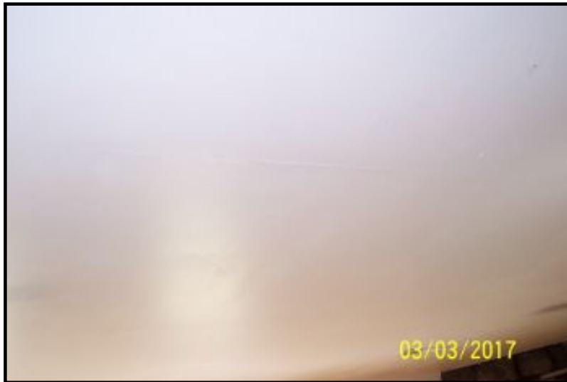
tape spiting in livingroom most likely settling
