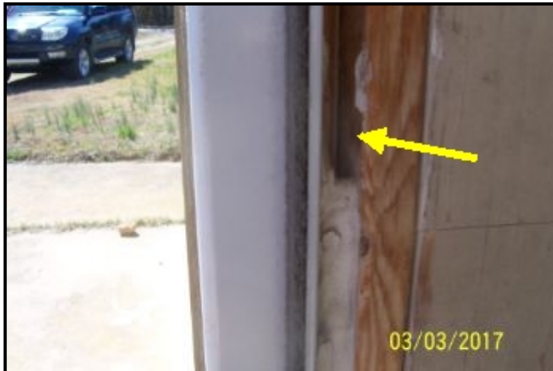
right side door jam needs caulking
