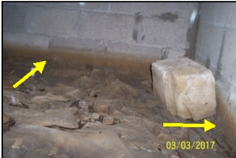
prior water drainage marks, may be gutter issue
