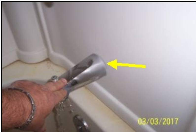
faucet somewhat loose to wall
