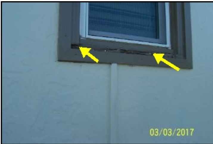
window sill shows signs of decay, replace
