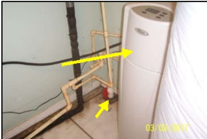
main water cut-off, water filter system
