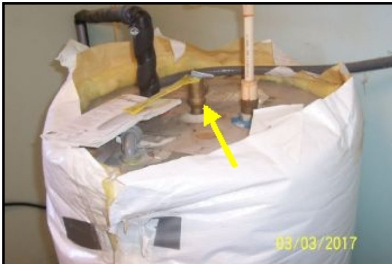
no overflow pipe
