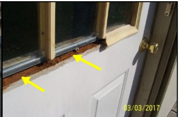
front door window seal deteriorated
