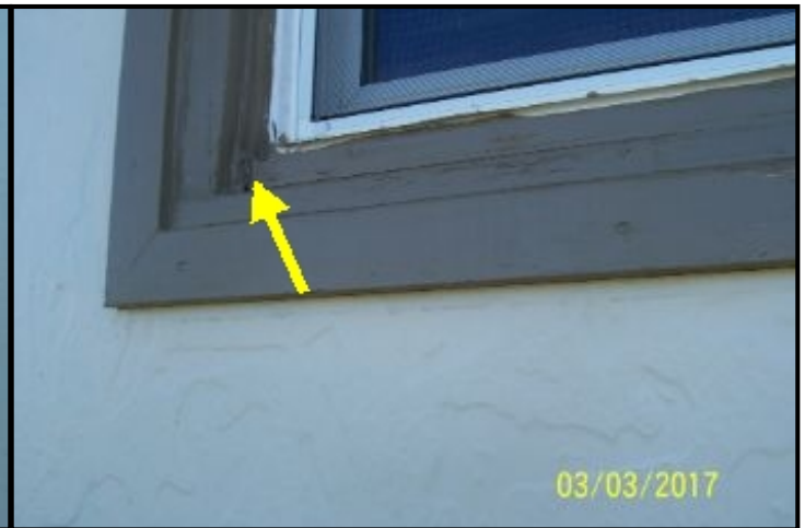
left side water damage
