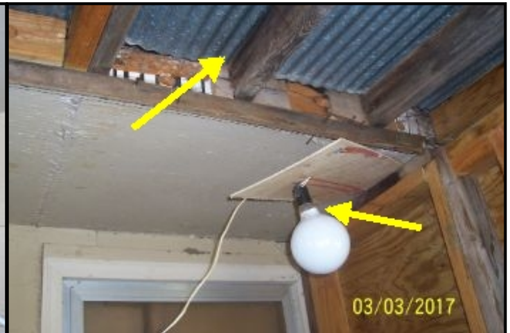
sunroom ceiling not finished, light hanging?
