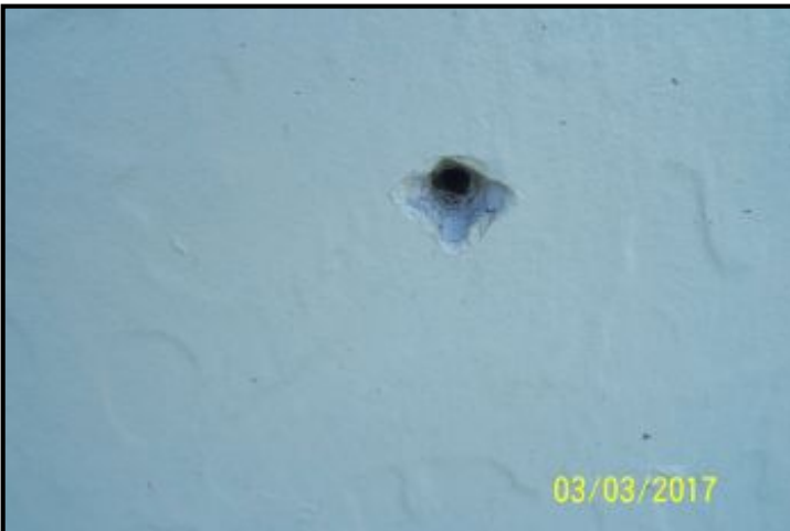
hole in siding needs filled
