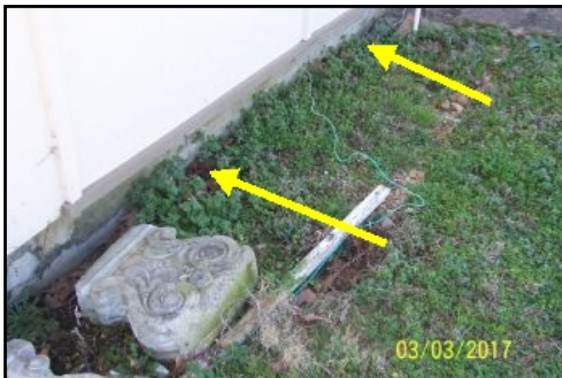
water needs to drain away from house
