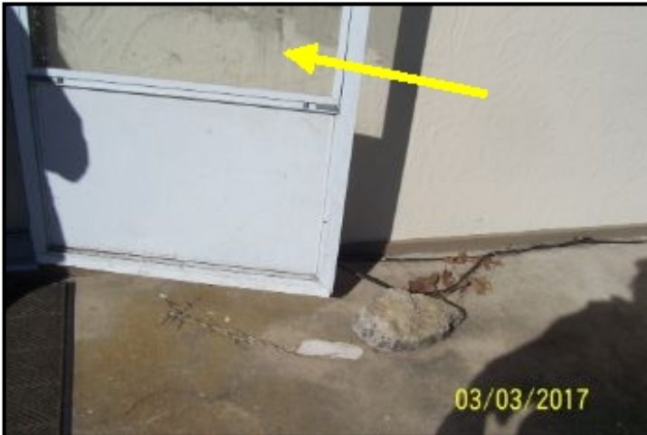
right side screen door does not automatically close, torn screen
