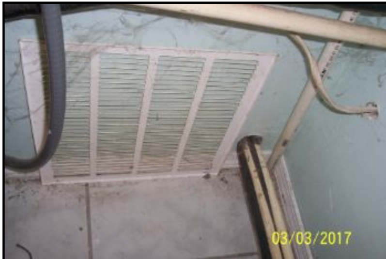
return air vent
