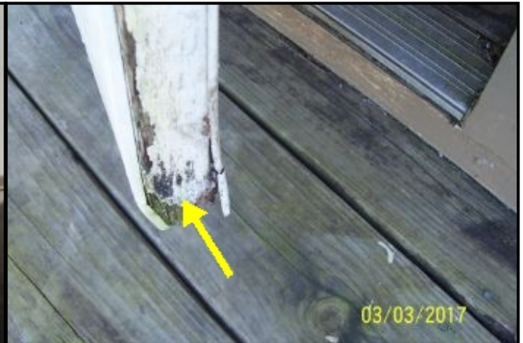
rear door shows water damage
