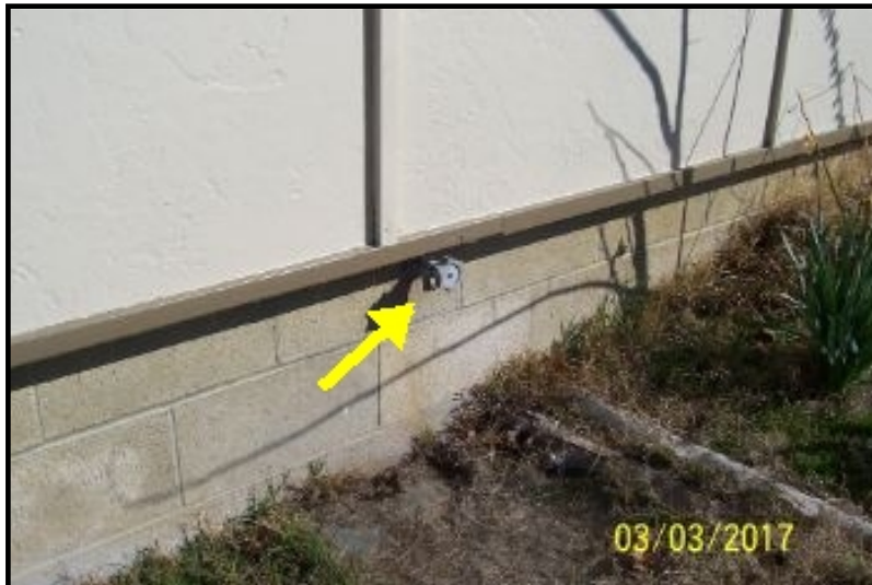
front did not operate properly
