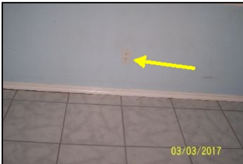
No ARC fault protection
