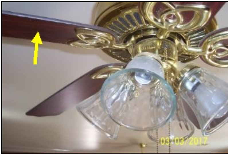
fan did not operate properly
