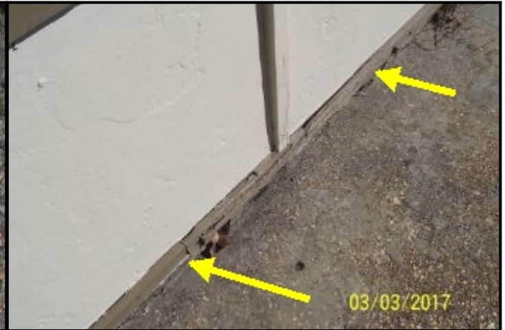
wood near concrete showing signs of deterioration, seal
