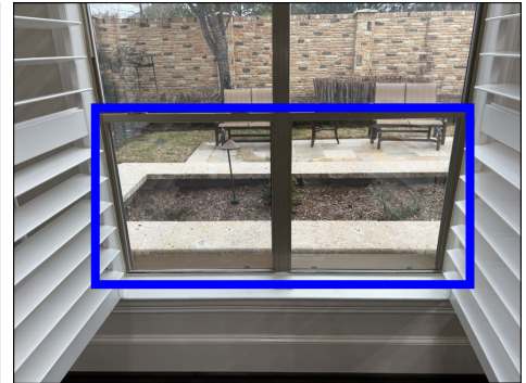
The window did not stay open when tested. Mainly at - Den (Main House)
