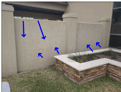
Minor cracks in stucco, recommend sealing with an acrylic paint. Mainly at - rear courtyard
