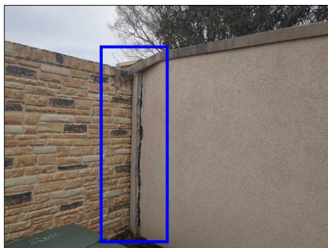
Although fences are not inspected it was noted that the stucco fence is showing some signs of damage or deterioration. right side
