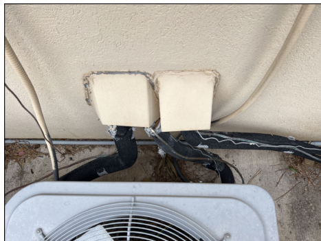
The insulation is missing or damaged on the A/C suction line at the condensing unit. Recommend repair or replacement to prevent cooling loss from exterior temperatures.
