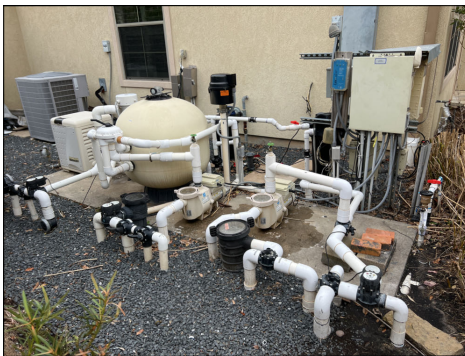
Overview of pool equipment
