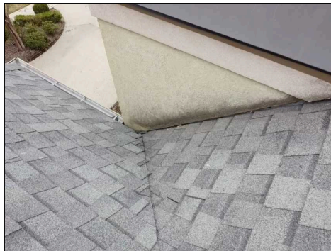
The stucco siding on the home is stained. Mainly at - front
