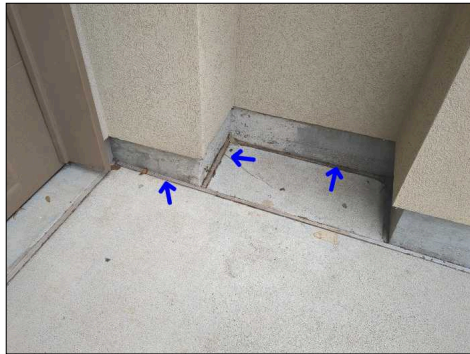
There are form boards noted at the slab, it is recommended that all form boards be removed from around the slab to help prevent conducive conditions for wood destroying insects as deteriorating wood is a conducive condition for wood destroying insects. Mainly at - guest house
