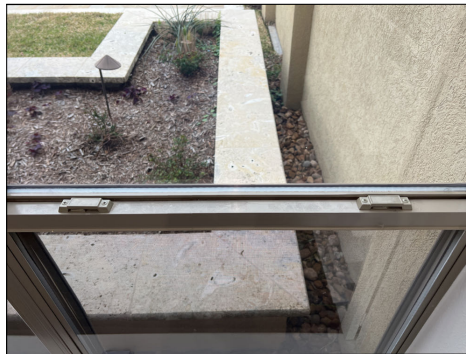
The window lock/latch is missing/broken. Mainly at - Den
