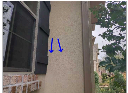
Minor cracks in stucco, recommend sealing with an acrylic paint. Mainly at - front of the guest house
