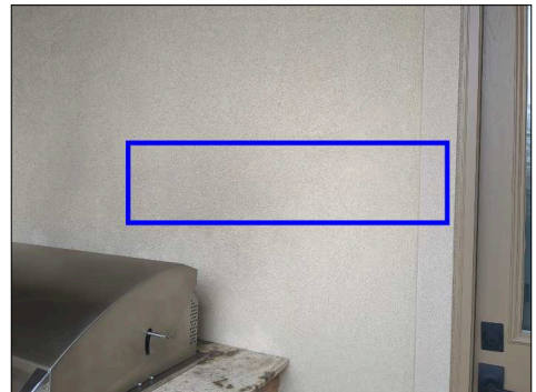
Minor cracks in stucco, recommend sealing with an acrylic paint. Mainly at - rear left of guest house
