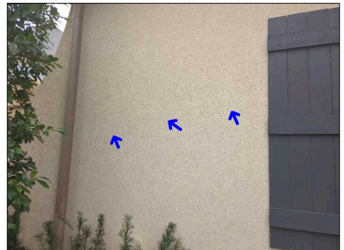
Minor cracks in stucco, recommend sealing with an acrylic paint. Mainly at - front left of guest house
