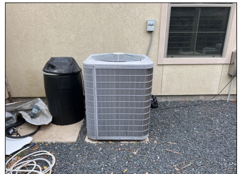
Overview of A/C Condenser (Guest House)
