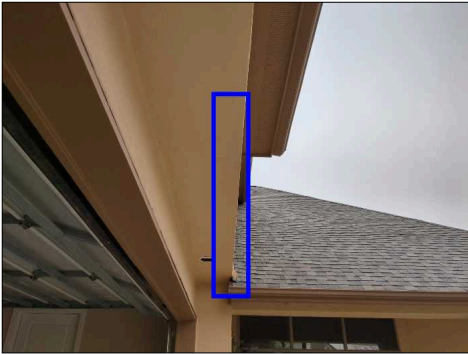
The stucco wall is missing the weepscreen at the bottom of the wall. It is recommended that water have a way to exit from behind the wall to help prevent deterioration of the substrate behind the stucco.
