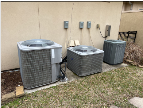
Overview of outside A/C units for the main house
