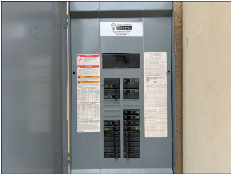
Overview of main electrical panel
