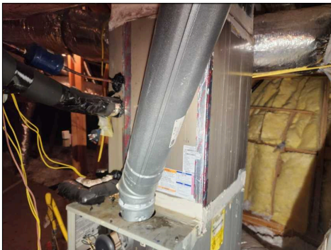
Overview of A/C Evaporator (Unit #2)
