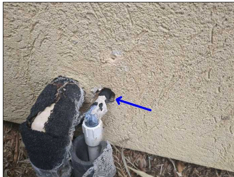
Recommend sealing gaps & holes in stucco to help prevent water penetration. Mainly at - front left of guest house
