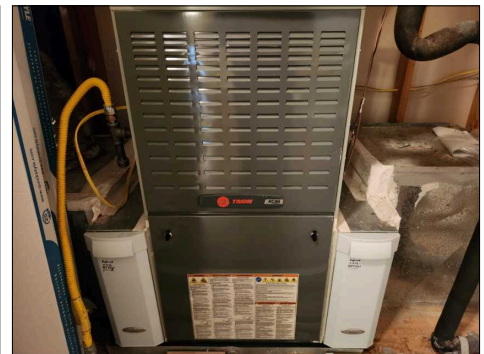
Overview of Furnace equipment (Unit #4)
