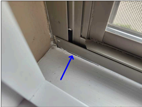
Sealant is needed around the interior of the windows between the window framing and the drywall to help prevent water penetration. Mainly at - Guest house front entryway
