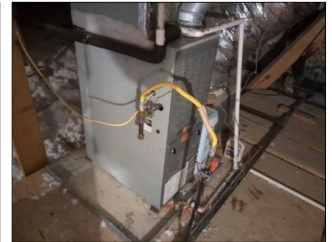
Overview of Furnace equipment (Unit #3)
