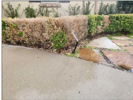
Head(s) is at an angle limiting its spray pattern, recommend straightening head to reestablish proper spray. Zone - 7
