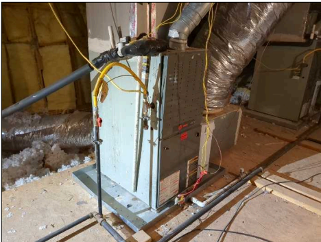
Overview of Furnace equipment unit #2. Trane
