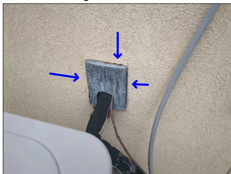
Recommend painting and sealing the A/C line entry cover at wall connection to help prevent deterioration and water penetration.
