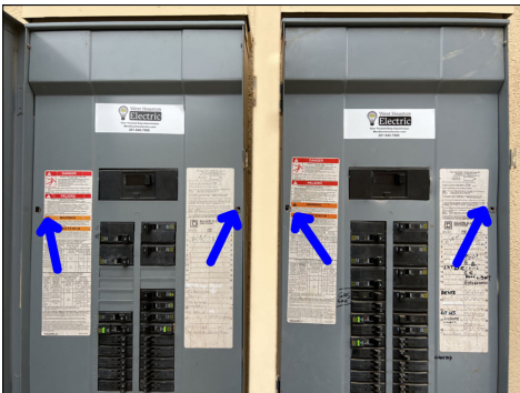
Panel cover is missing one or more screws.
