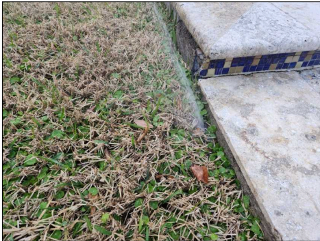
Head(s) are not popping up high enough to clear grass causing limited spray coverage. Zone - 12
