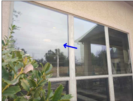
A hole was noted in a window pane. Mainly at - guest house rear
