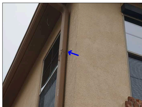
The gutter strap is damaged. Mainly at - left side
