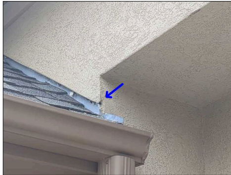
The improper kick-out / roof terminations need to have a proper flashing installed or the current flashing modified or replaced and sealed to prevent water intrusion through the system at these areas. During the installation of any flashing the immediate area can be inspected for wood rot or damage. Any other roof flashing in the area should also be checked as they sometimes can be a contributing cause. We suggest that the sidewall flashings of the roof be set in roof cement in the areas of kickouts as a preventative measure. Mainly at - left rear of guest house
