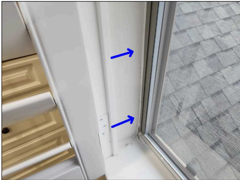
Sealant is needed around the interior of the windows between the window framing and the drywall to help prevent water penetration. Mainly at - main house upstairs game room
