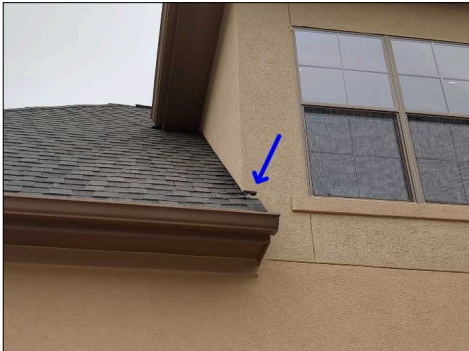
The roof is missing the kick out flashing at the end of the roof to sidewall connection. This is to help prevent water from running down or in the wall causing possible water penetration and deterioration. This is extremely important at stucco sidewall connections to help prevent water from penetrating behind the wall. Mainly at - right side main house
