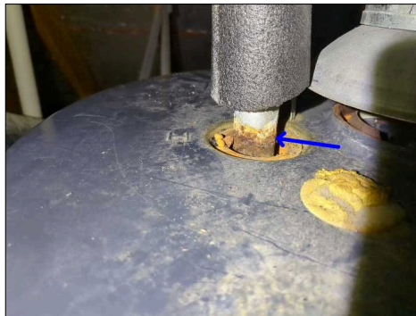
There are indications of electrolysis noted at the water heater supply fittings evident mainly by rust and corrosion. Left side unit
