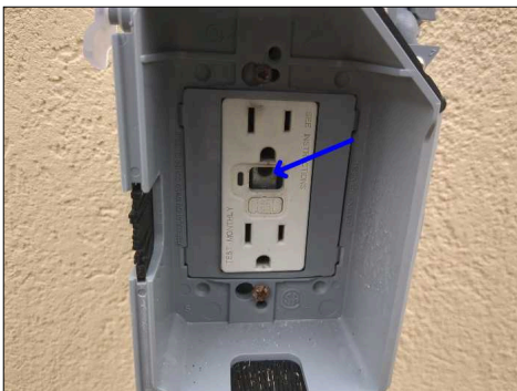
The GFCI (Ground Fault Circuit Interrupter) electrical outlet does not reset when tested and is showing no power. Mainly at - left side of main house
