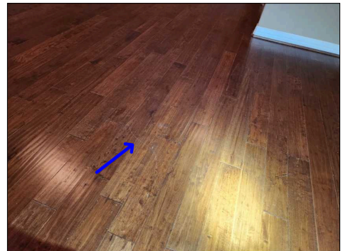
There are scratches noted in the wood flooring. Mainly at - guest house gameroom
