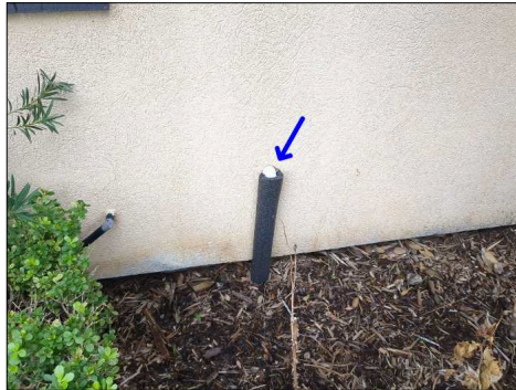
Recommend sealing gaps & holes in stucco to help prevent water penetration. Mainly at - front right of main house
