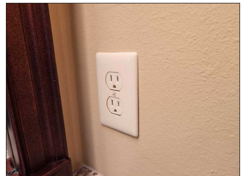
Switch plate is loose. Recommend securing to help prevent electrical shock. Mainly at - guest house 2nd floor bath
