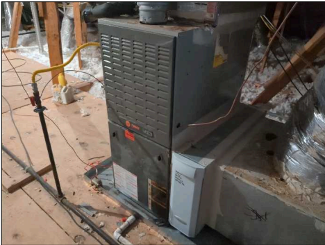
Overview of Furnace equipment unit #1. Trane
