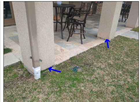
The patio post are showing signs of deterioration or damage recommend repairs or replacement to help prevent further deterioration.
