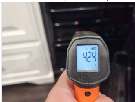
The bar or wine refrigerator is operating as intended. (Main House Upstairs Game Room)
