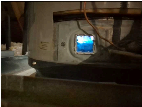
Overview of water heater burner compartment right side unit
