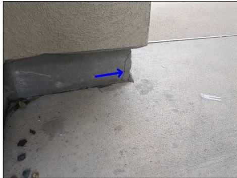
Corner pops were noted on one or more corners of the foundation, these are usually considered cosmetic nature unless other movement is noted. Recommend sealing all cracks to help prevent further deterioration.
