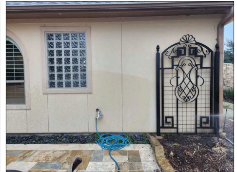
Recommend adjusting the sprinkler head by the home so that it does not spray the structure. Allowing the sprinkler to spray the home can cause water damage and/or penetration. Zone - 15
