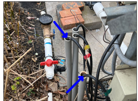
Silicone should be added to the conduit to help prevent water intrusion.
