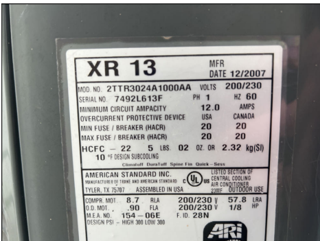
Overview of Condenser Manufacturers Tag (Right Unit) Trane, Dec. 2007
