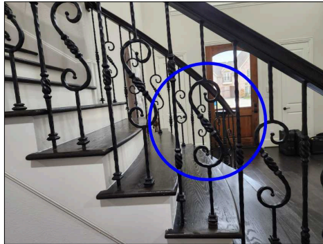
The rails on the stairway or balcony are climb able, this is a safety concern and it is recommended that all rails be installed in such a way that they cannot be climbed by children or pets.
