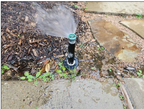
There is a broken sprinkler head. Zone - 7
