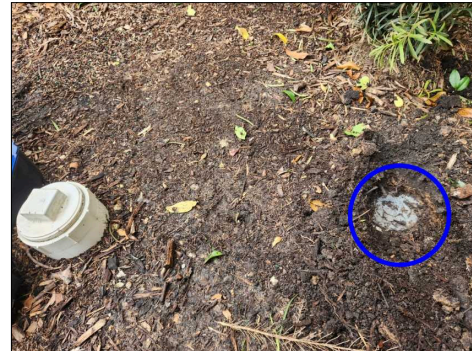
The height of the clean out is below the grade of the soil. It is recommended that the riser be elevated above grade to help identify entry points of the sewer line in the event that there is a need to gain access to the line to clear potential future blocks or obstructions. Mainly at - Guest House
