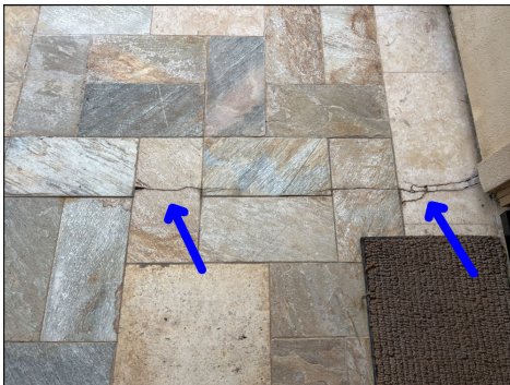
Cracks were noted in the tile, unable to determine the condition of the underlying surface. Mainly at - rear patio (main house)
