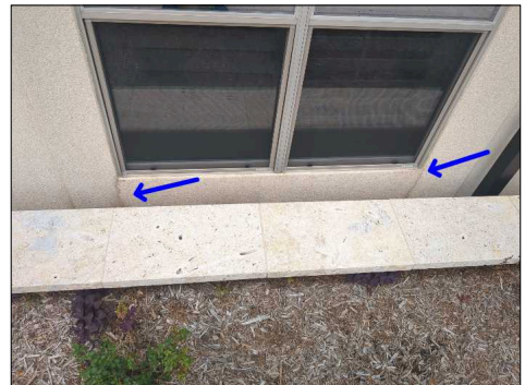
Minor cracks in stucco, recommend sealing with an acrylic paint. Mainly at - rear right of main house
