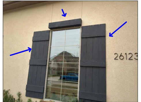
Recommend sealing gaps & holes in stucco to help prevent water penetration. Mainly at - front right of main house
