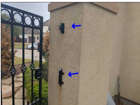
Recommend sealing gaps & holes in stucco to help prevent water penetration. Mainly at - guest house right side entry gate
