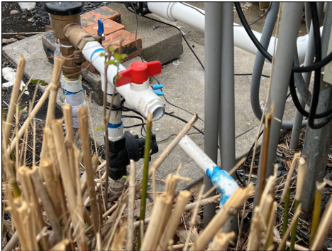
Water fill unit is disconnected.
