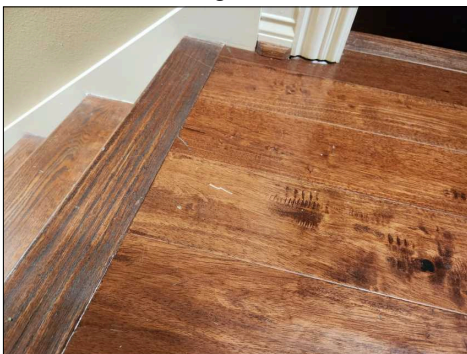
There are scratches noted in the wood flooring. Mainly at - guest house 2nd floor landing
