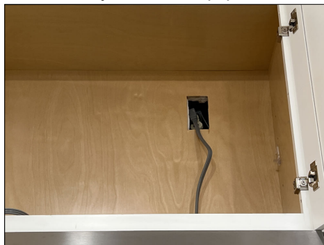
The electrical receptacle or box is loose, recommend securing and adding faceplate cover. Mainly at - Above vent hood in kitchen (Main House)
