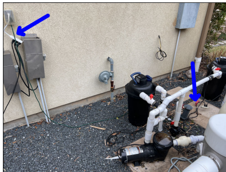
There is some extension cord type electrical wiring. Recommend wiring be replaced with permanent wiring. Mainly at - Pool Equipment
