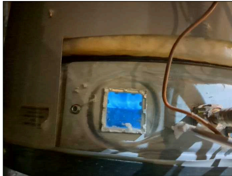
Overview of water heater burner compartment left side unit
