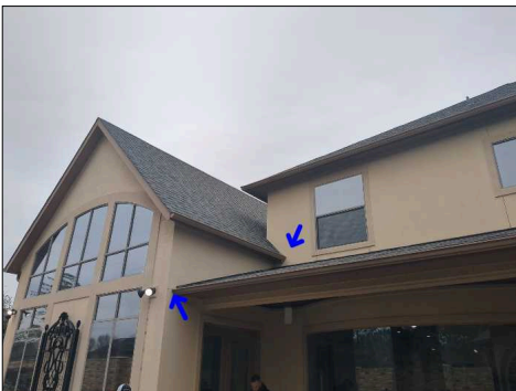
The roof is missing the kick out flashing at the end of the roof to sidewall connection. This is to help prevent water from running down or in the wall causing possible water penetration and deterioration. This is extremely important at stucco sidewall connections to help prevent water from penetrating behind the wall. Mainly at - patio of main house
