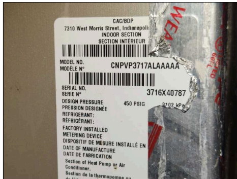
Overview of A/C Evaporator Manufacturers Tag (Unit #2) Trane, 37th Week of 2016
