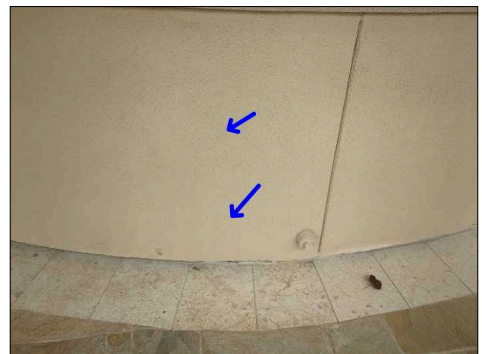
Minor cracks in stucco, recommend sealing with an acrylic paint. Mainly at - main house patio
