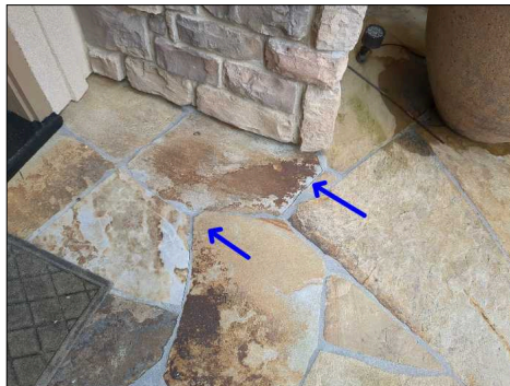
Minor settlement cracks are noted on the porch of main house
