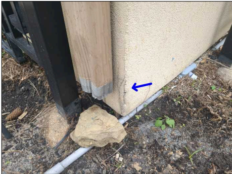
Stucco is damaged, recommend repairs to help prevent water penetration. Mainly at - rear left of main house
