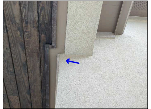
Minor cracks in stucco, recommend sealing with an acrylic paint. Mainly at - breezeway between homes
