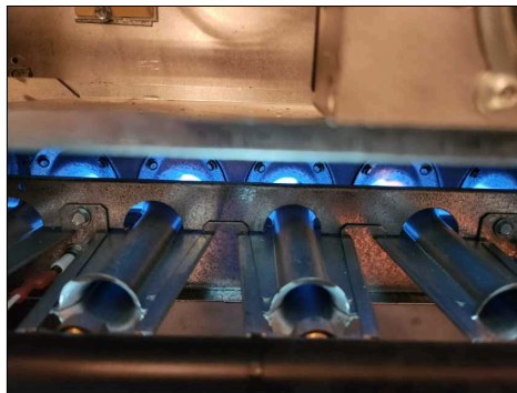
Overview of Furnace burner compartment. (Unit #4)
