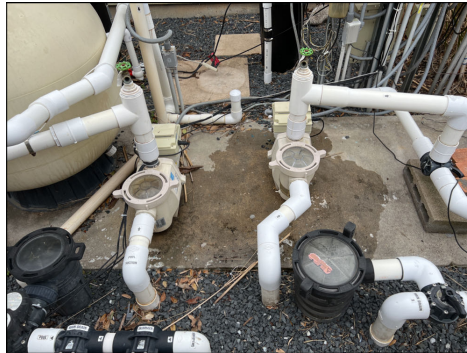
There is a water leak at the pool equipment. Mainly at - unable to determine location of leak
