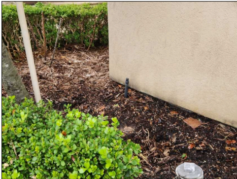
There is low pressure at the spray heads. Zone - 2
