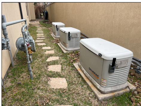
There are (3) backup generators installed on the property. Generators are not part of a normal home inspection therefore they were not inspected. Recommend contacting a licensed electrician for full evaluation of generator systems.
