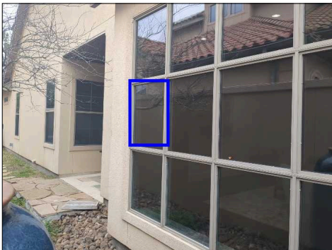
Window pane(s) have lost their thermal seal. Signs of lost seals in the thermal pane windows may appear and disappear as temperature and humidity changes. Recommend having a window contractor check all windows for lost thermal seals as all windows may not be noted. Mainly at - left side of main house
