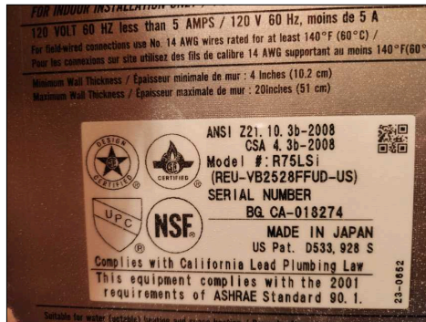
Overview of Water Heater Manufacturers Tag (Guest House) Rinnai, Nov. 2010
