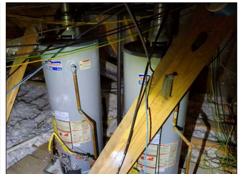
Overview of Water Heaters (Main House)
