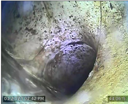
Sewer lateral connection from guest house to main house drain line @ 44 ft.
