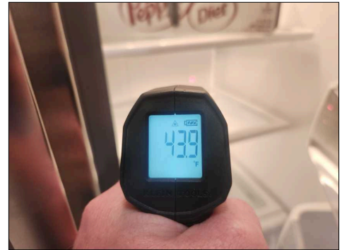
The refrigerator is operating as intended. (Guest house)
