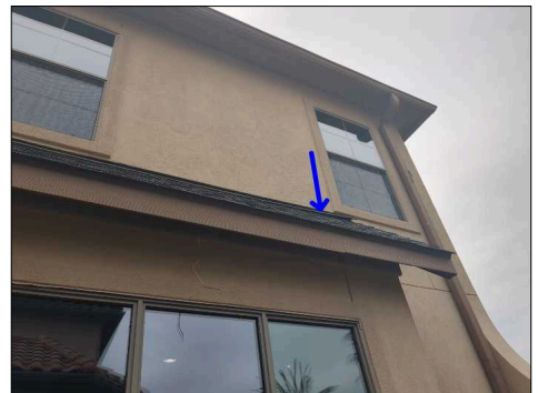
The roof flashing is lifted. Recommend securing all loose or lifted flashing and sealing nails to help prevent water penetration. Mainly at - left side of main house
