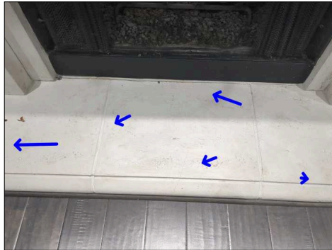
Settlement cracks are noted in the hearth, recommend sealing. Left front fireplace
