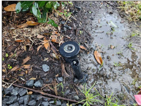
There is a broken sprinkler head. Zone - 12
