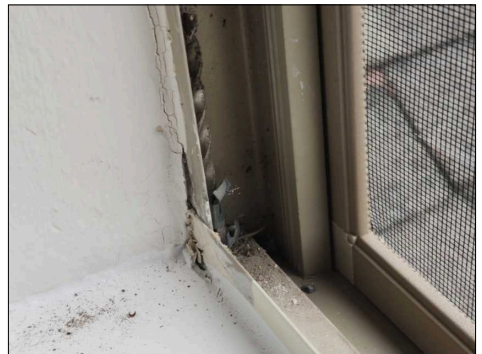
Springs were not attached or broken on window(s). Mainly at - Upstairs Game Room (Main House)
