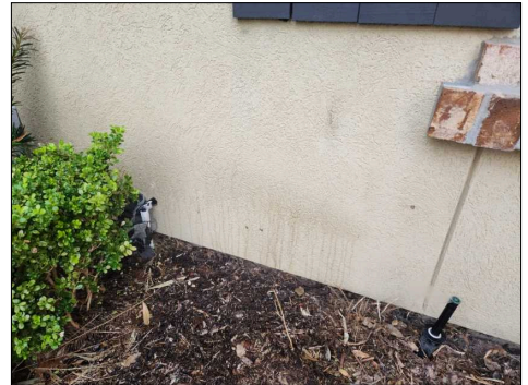
Recommend adjusting the sprinkler head by the home so that it does not spray the structure. Allowing the sprinkler to spray the home can cause water damage and/or penetration. Zone - 7
