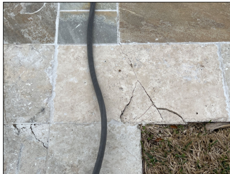
Tiles are chipped and/or cracked. Mainly at - throughout pool deck surround
