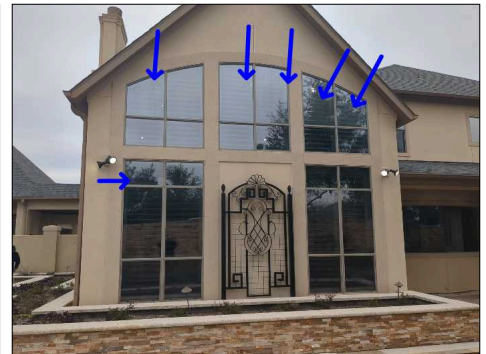
Window pane(s) have lost their thermal seal. Signs of lost seals in the thermal pane windows may appear and disappear as temperature and humidity changes. Recommend having a window contractor check all windows for lost thermal seals as all windows may not be noted. Mainly at - rear right side main house
