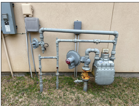
Overview of Gas delivery manifold.
