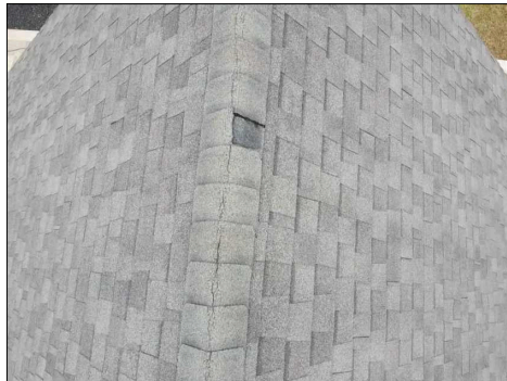
There are damaged or missing ridge shingles on the roof, recommend repairs or replacement of damaged ridge shingles.
