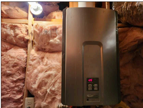
Overview of water heater (Guest house)
