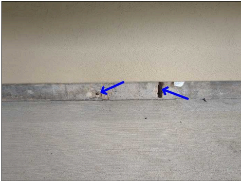
One or more of the post tension cables were noted to be exposed, recommend using a rust inhibitor to all rusting cables and sealing all exposed post tension cables noted around the foundation of the house to help prevent premature deterioration of the post tension cables.
