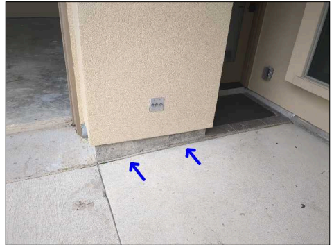
There are form boards noted at the slab, it is recommended that all form boards be removed from around the slab to help prevent conducive conditions for wood destroying insects as deteriorating wood is a conducive condition for wood destroying insects. Mainly at - main house
