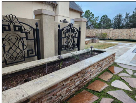
The heads or hoses of the drip system were exposed above grade. The drip system is intended to be buried as it is a direct source for watering a tree or shrubs root system. Recommend burying the components below the soil to help promote better watering and coverage. Zone - 17
