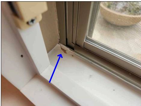
The window sill is peeling due to condensation moisture damage, recommend repairs to help prevent further deterioration. Mainly at - guest house living room
