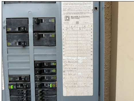
The breakers in the main electrical panel are partially labeled.
