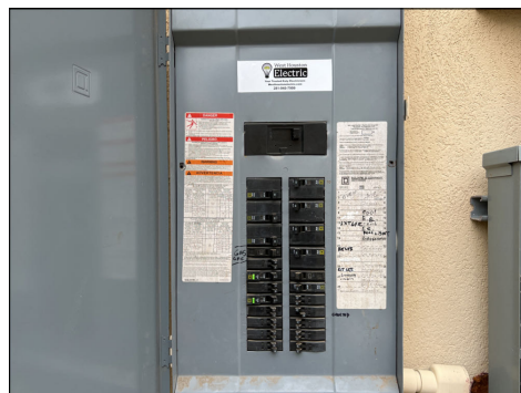
Overview of main electrical panel
