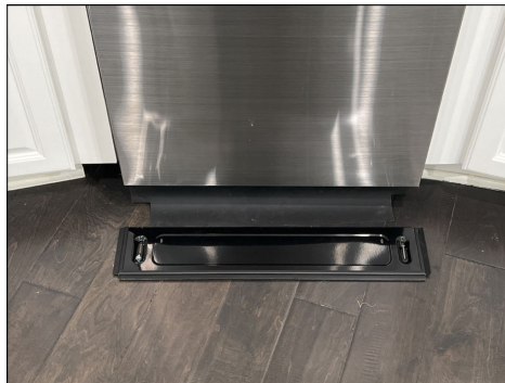
The kick plate is not installed on the dishwasher. (Main House)
