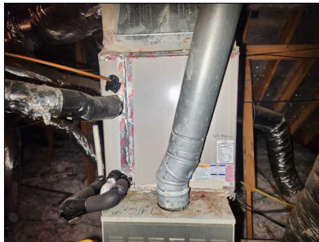
Overview of A/C Evaporator (Unit #1)
