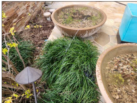
The heads or hoses of the drip system were exposed above grade. The drip system is intended to be buried as it is a direct source for watering a tree or shrubs root system. Recommend burying the components below the soil to help promote better watering and coverage. Zone - 8
