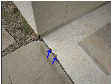
Damage was noted in the stonework. Recommend sealing to help prevent further deterioration. Mainly at - main house left side patio
