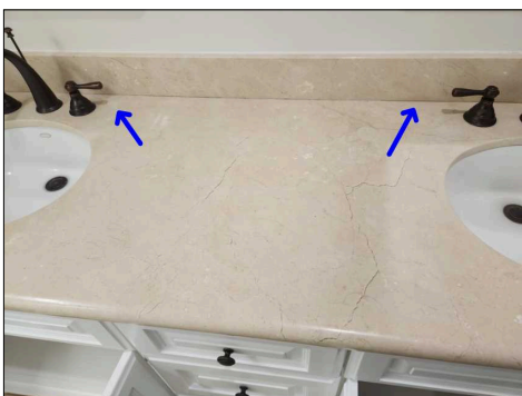
Seal countertop at wall connection. Mainly at - Upstairs Left Front Bath (Main House)
