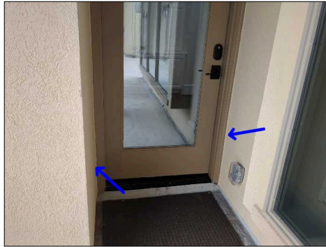
Recommend sealing between the trim and stucco to help prevent water penetration. Mainly at - main house right side door
