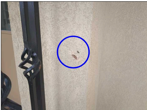
Recommend sealing chips in stucco to help prevent water penetration. Mainly at - right side of driveway pool entrance
