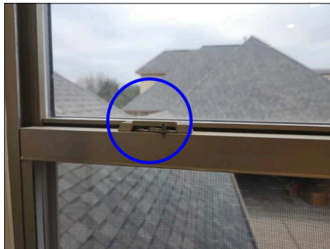
The window lock/latch is damaged. Mainly at - Upstairs Game Room (Main House)
