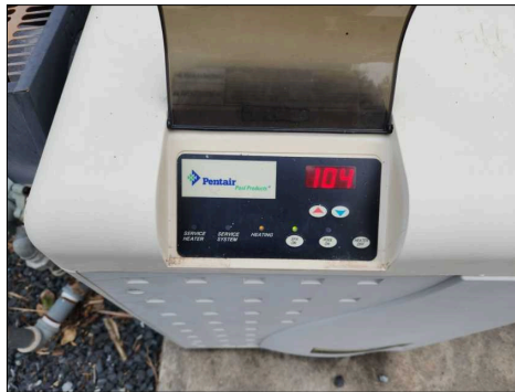
Overview of pool heater
