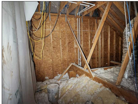
The insulation for the exterior wall is missing. Recommend replacing missing insulation for proper energy efficiency. Mainly at- Upstairs Left Rear (Main House)
