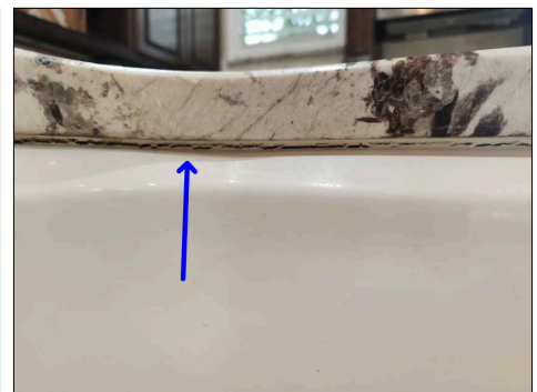
Undermounted sinks require sealant between the sink and counter top to help prevent water penetration to the surfaces below. Recommend sealing or repairing seal to help prevent water penetration and potential moisture damage to the underlying materials. Mainly at - guest house kitchen
