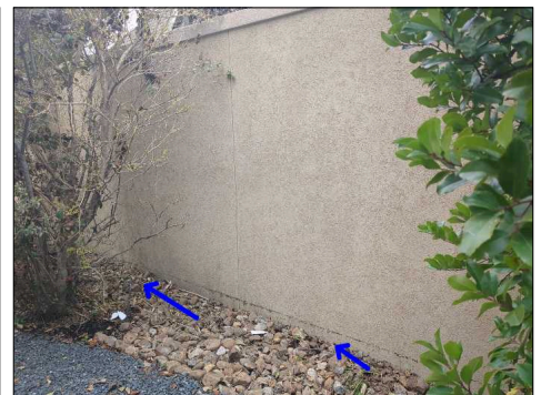
Recommend having a 4 to 6 inch gap between a stucco and grade to help prevent the system from wicking moisture up and causing possible feature damage. right side
