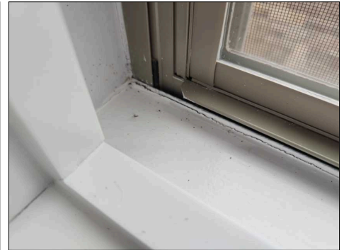
Sealant is needed around the interior of the windows between the window framing and the drywall to help prevent water penetration. Mainly at - Guest house master bedroom
