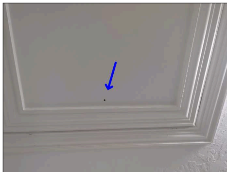
The pull down attic ladder is missing the pull string. Recommend installing a new pull string or an eye hook for access to the attic. Mainly at - Main Attic (Main House)
