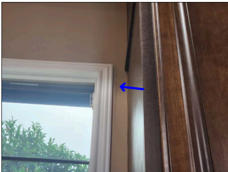
Settlement cracks were noted in the drywall. Mainly at - guest kitchen
