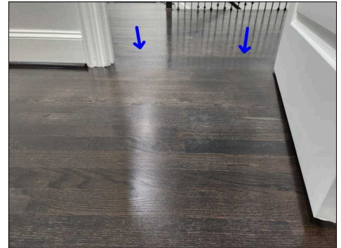
Uneven or sloping floors were noted. Some times in older homes minor slopes may be due to construction methods at that time, however if floors are sloping more than normal it is recommended that some follow up investigation be made. Sloping floors can be caused by foundation movement or from structural issues usually on upper floors. Floors were noted to be sloped. Mainly at - Upstairs Right Rear Bedroom (Main House)
