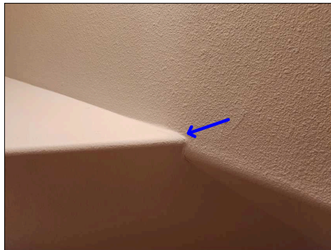
Settlement cracks were noted in the drywall. These are generally considered cosmetic only, unless otherwise noted. Mainly at - guest house gameroom
