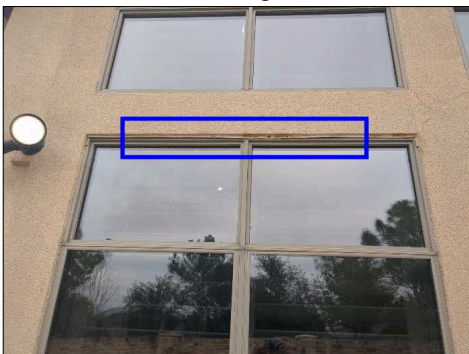
The flashing details are showing signs of rust / deterioration. This is often caused by excess moisture. Recommend repairs and or replacement as needed.
