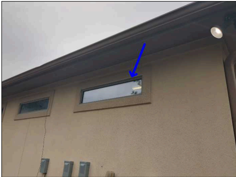
Window pane(s) have lost their thermal seal. Signs of lost seals in the thermal pane windows may appear and disappear as temperature and humidity changes. Recommend having a window contractor check all windows for lost thermal seals as all windows may not be noted. Mainly at - rear left of Maine house
