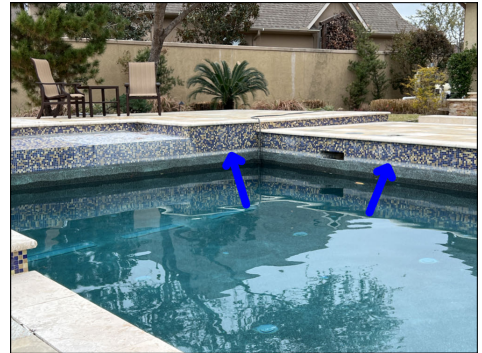
There are mineral stains on the pool walls and or surrounding equipment. Recommend a chemical analysis be performed on the pool water to verify safe water chemistry.
