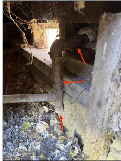
Rusted gas line
